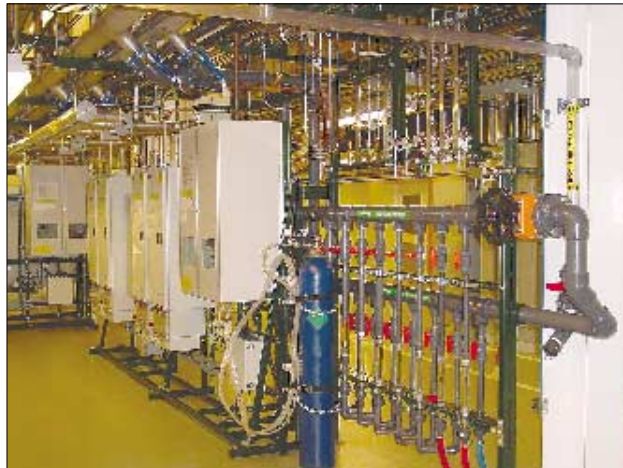
Safety is the primary focus for all gas handling facilities at the PMTC, which included the use of torque elimination fittings in process gas lines.
